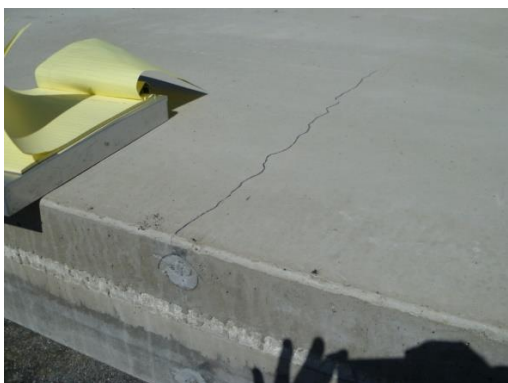
Figure 2.7 Top layer of longitudinal prestressing strand splitting failure
