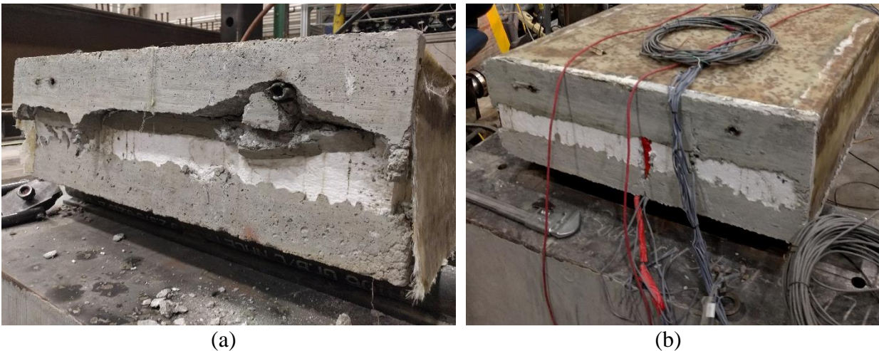
Figure 3.27 (a) Slip at the end of the south side, (b) No slip is detected at the north side
