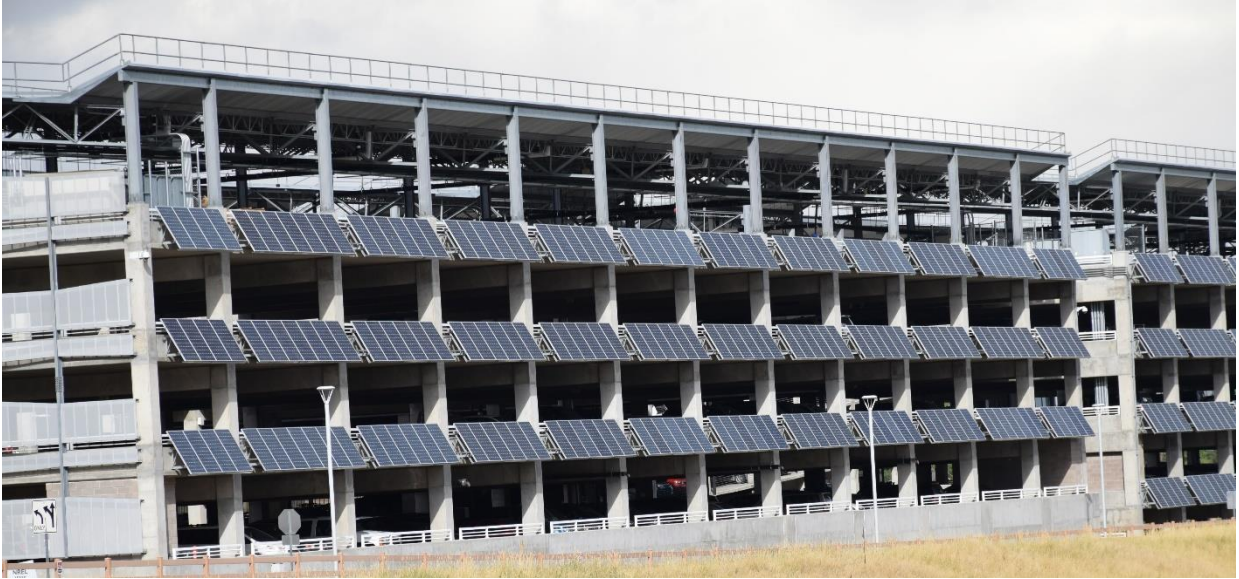
Figure 1.1 PV modules mounted to the wall of a multistory parking at NREL, CO
